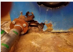
Picture #1 View of Boiler at Point of Failure
