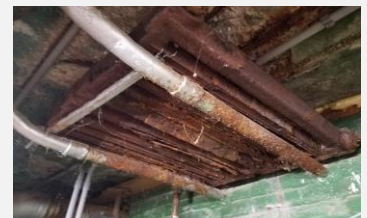
Picture #2 View of Ceiling Radiator Corrosion
